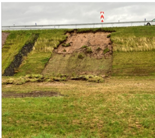
FIGURE 1. View of the site of interest with a collapsed slope.
