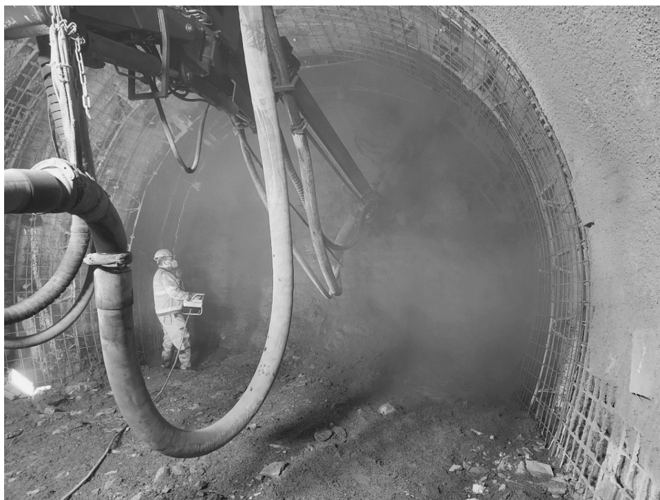
FIGURE 5. Spraying of first shotcrete layer in the new advance, while reinforcement with no concrete can be seen in the bench area of the previous advance.
