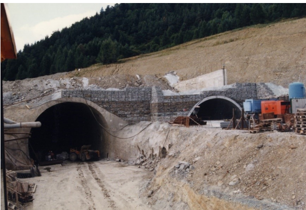
FIGURE 3. The eastern portal of the tunnel Branisko, left - monolithic, right - prefabricated shell structure (photo by Ing. Libor Mařík [2])
