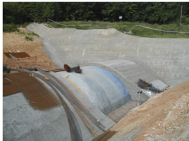
FIGURE 4. The shell structure on the Schellenberg tunnel (photo by Ing. Jiří Zmítko)
