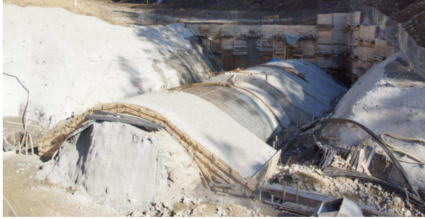
FIGURE 5. The shell structure supported by micropiles in the central pit of the tunnel Považský Chlmec (photo by Ing. Libor Mařík [2])
