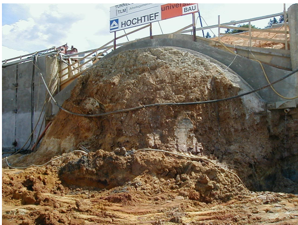
FIGURE 6. The fixed shell structure on the Euerwang tunnel (photo by Ing. Jiří Zmítko)
