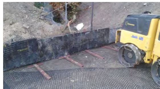
FIGURE 4. Formwork for proper compaction of reinforced soil structure with wrap-around facing in the facing area.
