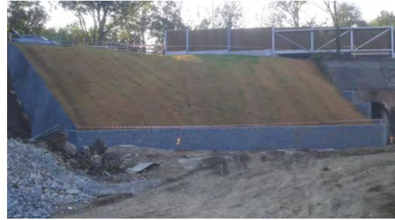
FIGURE 7. Overall view on the finished reclaimed slope, where grassing can be seen
