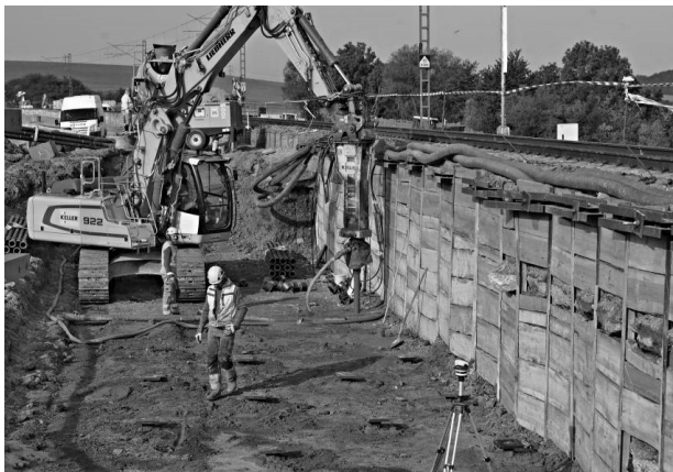
FIGURE 5. Stone columns procedure under the track no. 1. (top) and procedure of the Ductile piles under the track no. 1 (bottom).
