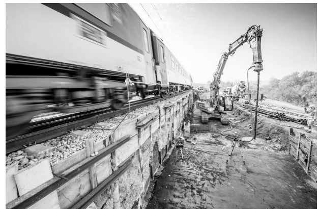
FIGURE 7. Vibro-stone columns and excavation for ductile piles under the track no. 2 (top) and ductile piles hammering under the track no. 2 (bottom).
