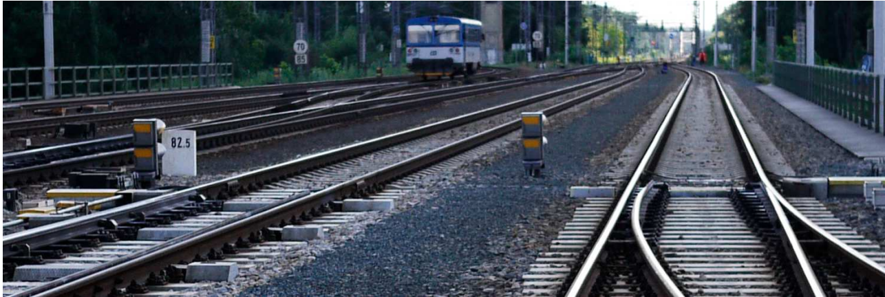
FIGURE 3. View of the track on the bridge in the direction from fixed bearing.
