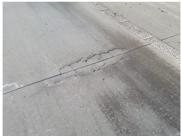
FIGURE 9. Damage to the cement concrete pavement at the transverse joint of the D5 motorway.
