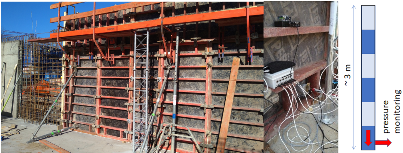
FIGURE 3. View on wall formwork (left), instrumentation at the bottom of the wall (middle), schematics of the wall cross section and position of built-in pressure sensors (right).
