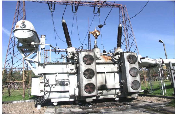
Fig. 2. Damaged bushing 220 kV in the 160 MVA power transformer
