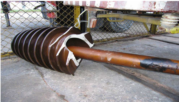
Fig. 1. Damaged bushing 110 kV in the 70 MVA power transformer
