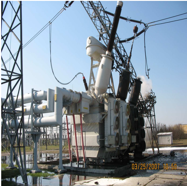
Fig. 2. Damaged bushings 400 kV in the 250 MVA power transformer
