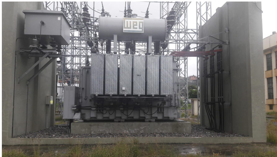
FIGURE 1. Picture of the 30/40 MVA, 138/13.8 kV Power Transformer studied in this work.
