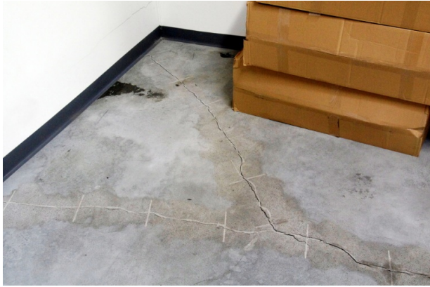
FIGURE 1. Cracks in the reinforced concrete floor of the hall in the corner near the cladding.
