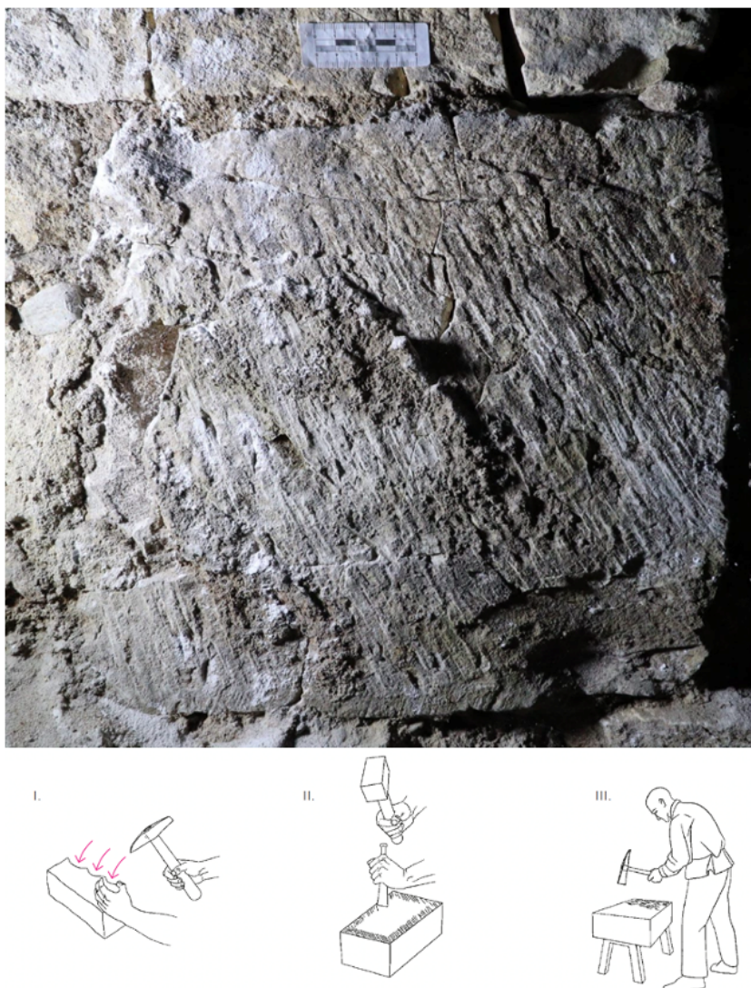
FIGURE 3. Old Town – Old Town Walls, between 1230 and 1253. Above, photo by M. Cihla, individual stages of working (drawing by A. Musilová, adapted from [13]).
