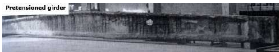
c) The fire damaged girder
