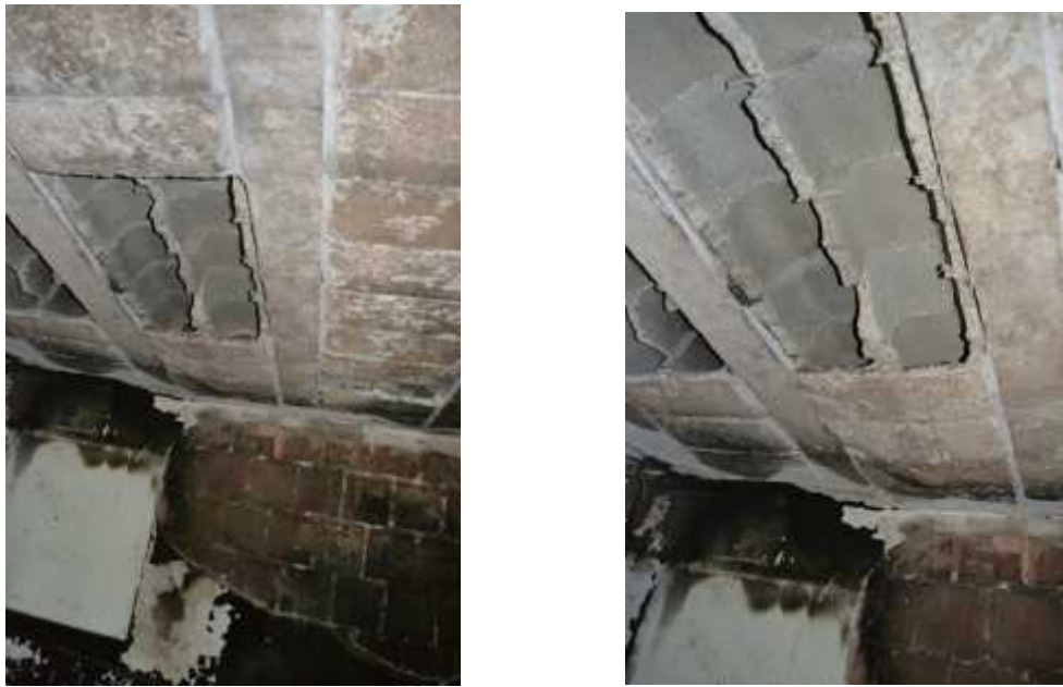
Fig. 8 The fire damaged girder-slab with concrete interjoists
