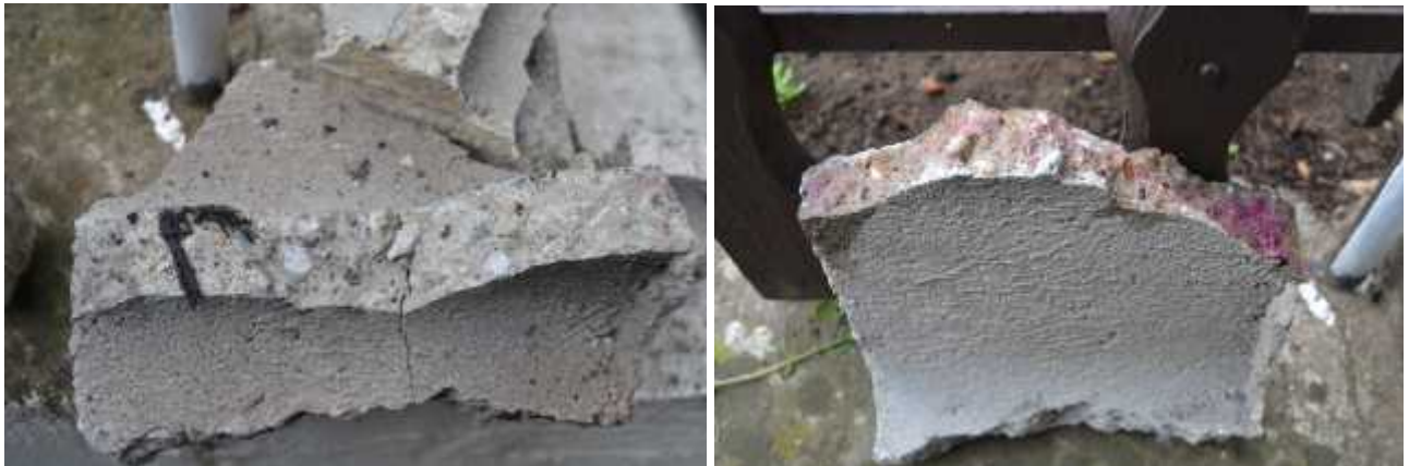
Fig 9. The fire damaged concrete interjoists
