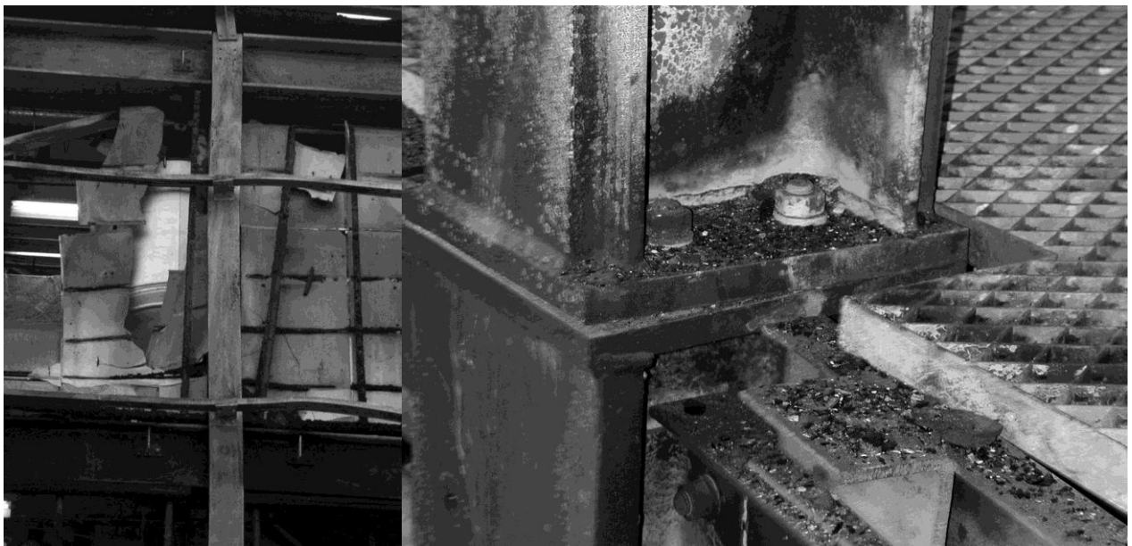
Fig. 1 Column with connecting members (left) and column base after fire damage in a production building
