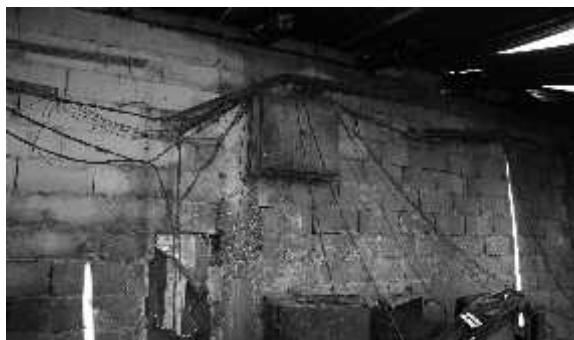
Fig. 4 Metal channels with cables
