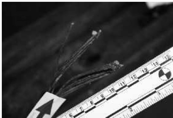
Fig. 3 Traces of melting wires at the place of break
