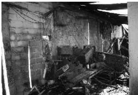
Fig. 1 Electrical installation in the burned room
