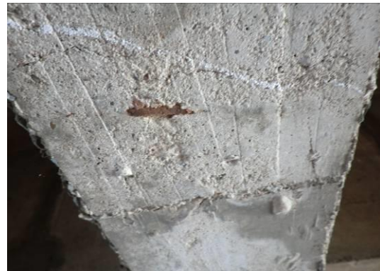
(b) - Concrete deterioration
