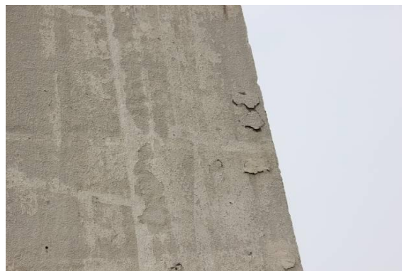
Fig. 6 - Concrete Damage in Sota (2)
