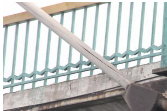
Fig. 4 - Anchor head protective cover fallen off
