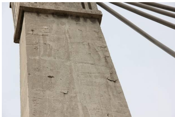
Fig. 5 - Concrete Damage in Sota (1)
