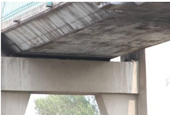
Fig. 3 - Rusting condition of steel main beam
