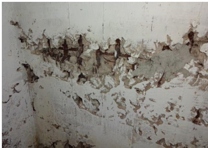
Fig. 6 – Visible cavities and reinforcement corrosion in the concrete structure
