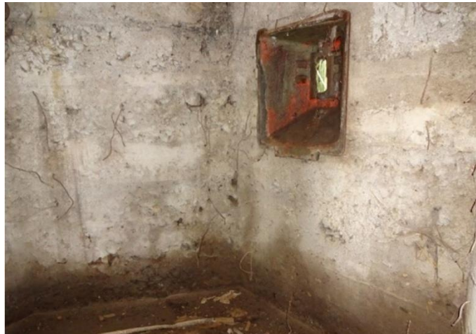
Fig. 5 – Moisture damage and visible cavities in the concrete structure
