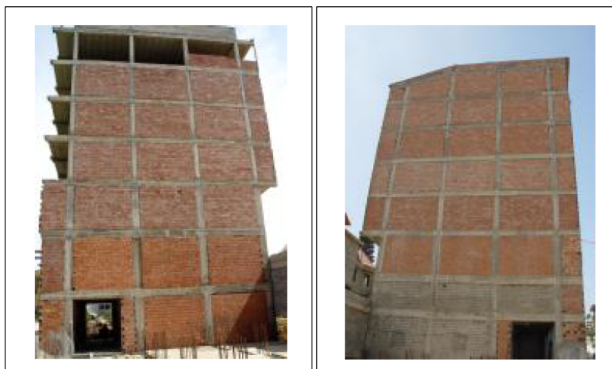
Fig. 2 – Chained masonry, BOUMERDES earthquake of May 21, 2003
