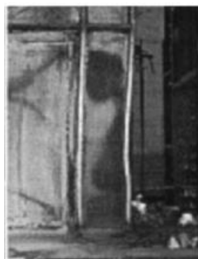
Fig .6 - yielding of the first floor column in the experiment [10]
