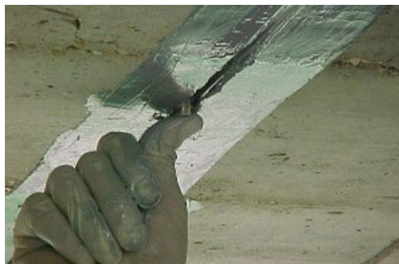
Fig. 2 – Use of FRP composites in surface grooves of a beam by the NSM method
