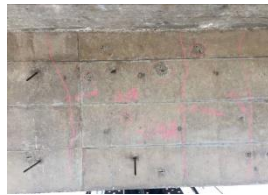
Vertical cracks in main span
