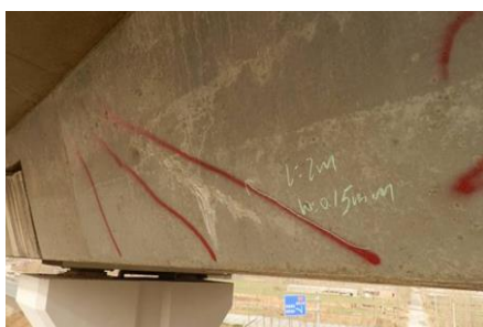
Fig. 2 – Diagonal cracks in web
