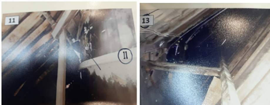
Fig. 2 - Damage to the roof frame of the Jakarta Sion Church.
