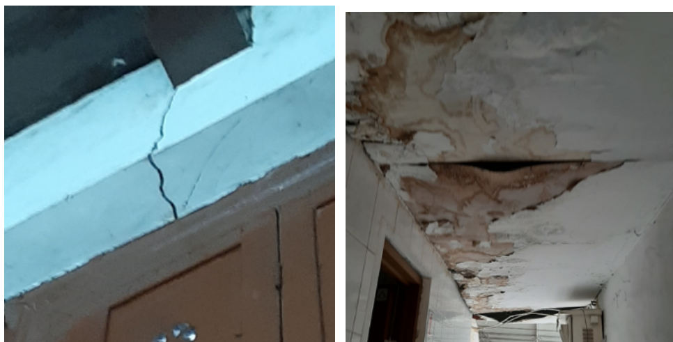
Fig. 4 - Cracked wall pairs (left) and damaged ceiling (right).
