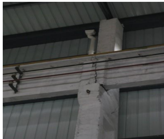
(h) Vertical cracking failure of crane beam
