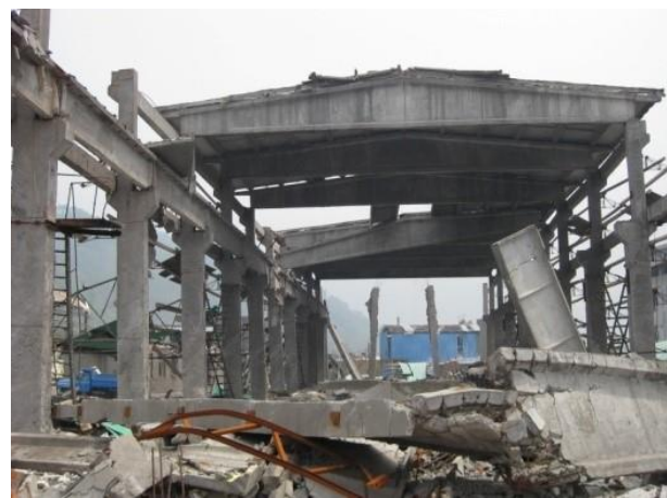
(d) Failure of roof slabs and beams in an industrial building
