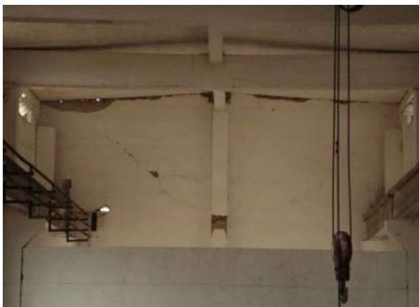
(c) Cracking of inner wall
