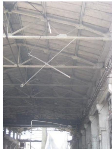
(b) Failure of horizontal contact
