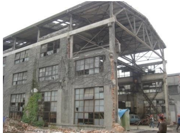
(b) Local collapse of building a wall of RC bent workshop
