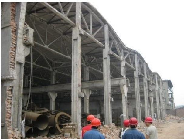
(c) Overall wall failure of maintenance wall
