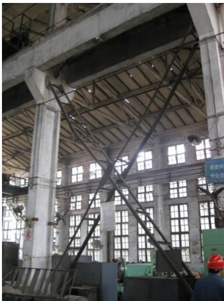
(a) Buckling of X-brace
