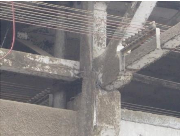
(e) Cracking and failure of corbel root
