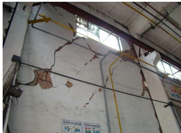
(b) Oblique cracking of wall
