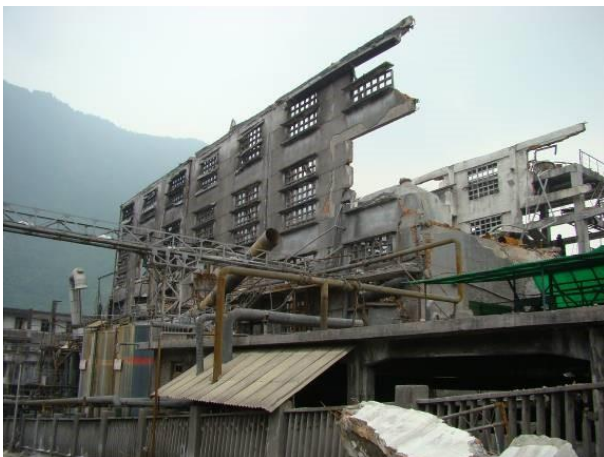
(a) Local collapse of RC industrial building
