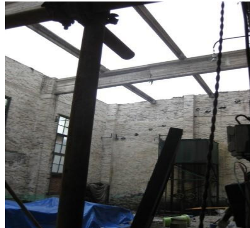
(f) Failure of upper transverse beam and plate of industrial building
