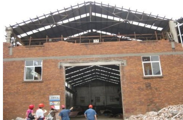
(f) Partial failure of upper maintenance wall
