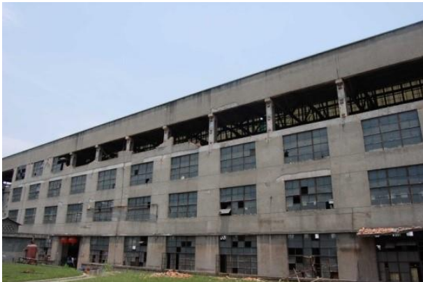
(e) Collapse of upper maintenance wall
