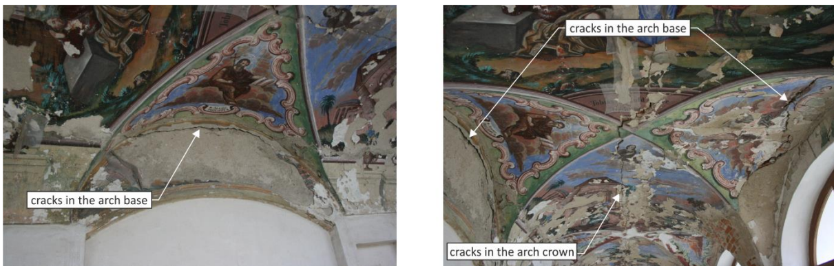
Fig. 7 – Examples of the failure of a barrel masonry vault with vaulted openings and cross vault of a historic building (Loretto near Bor u Tachova, West Bohemia, Czech Republic, 17th cent.)
