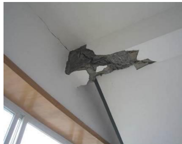
Fig. 5 – Failure of frame beams end
