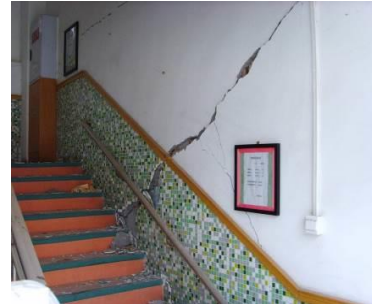
Fig. 9 – Cracking of staircase wall
