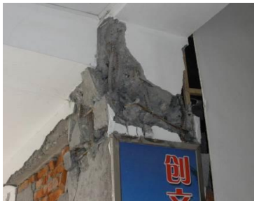
Fig. 4 – Failure of frame beams and columns
