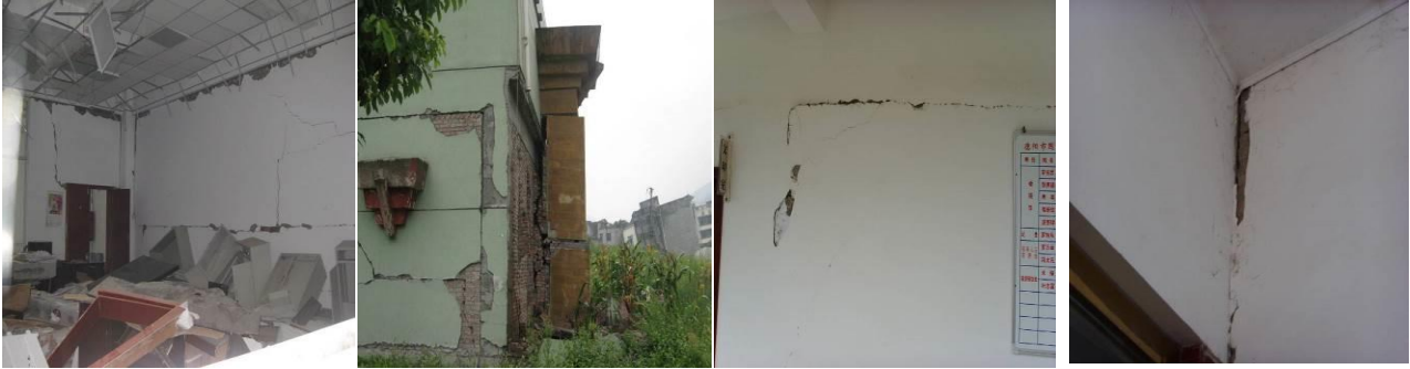
Fig. 1 – Cracks around filling wall
