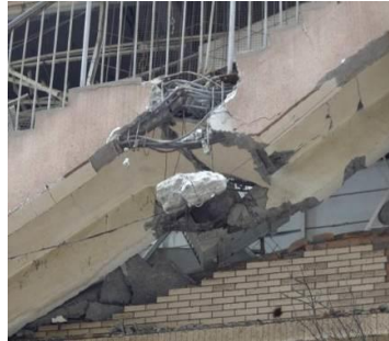
Fig. 8 – Stairboard midspan breakage and failure
