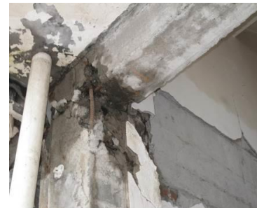
Fig. 6 – Failure of joint
