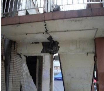
Fig. 7 – Fracture of stair platform beam
