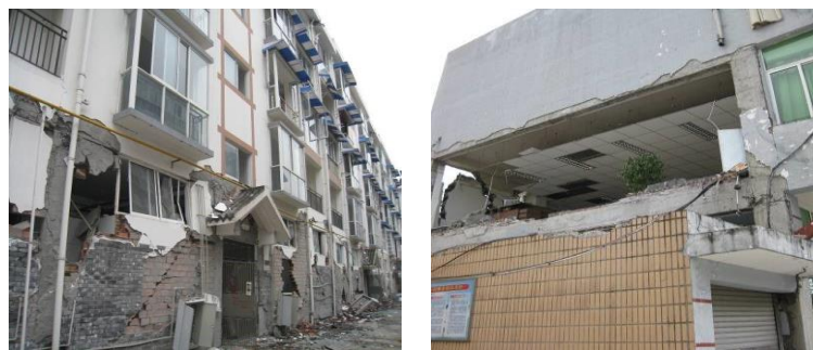
(a) Partial collapse of bottom filling wall
