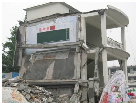
(a) Partial collapse
