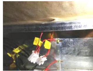
(f) – Separation of straw board and steel beam
