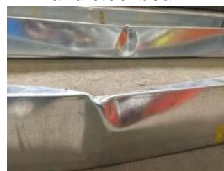
(h) – Buckling failure details of steel beam-A and beam-B
