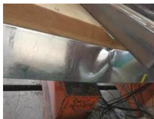
(c) – Local buckling of steel beam-A
