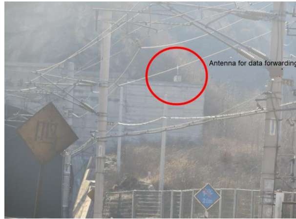
(b) Antenna for data forwarding at the tunnel exit
