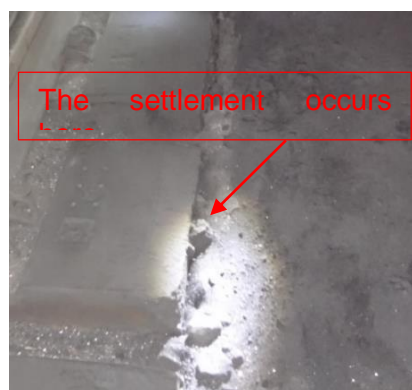
(a) Settlement of substructure
