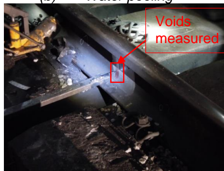
(c) Measurement of the underground voids
