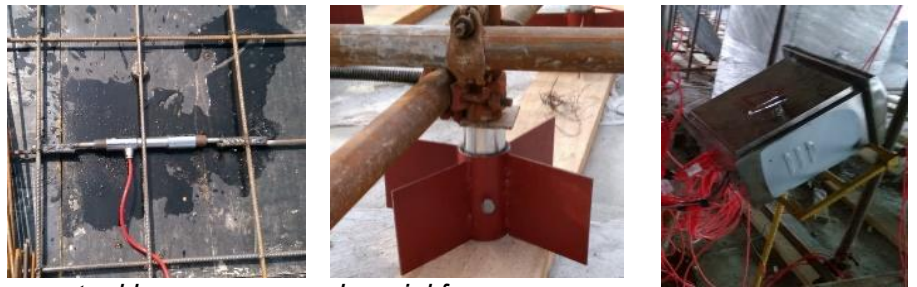
a. steel bar sensors installation b. axial force sensors installation c. acquisition system Fig.3 – Installation of sensors and acquisition equipment
