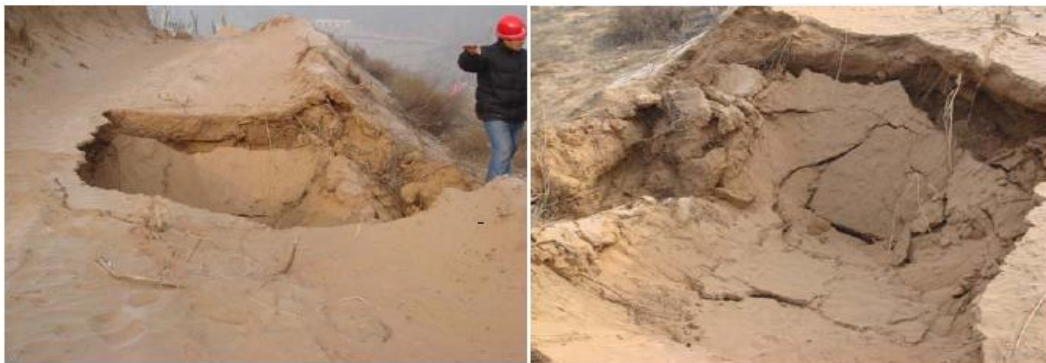
Fig.7 - Surface sandy land in tunnel exit section
