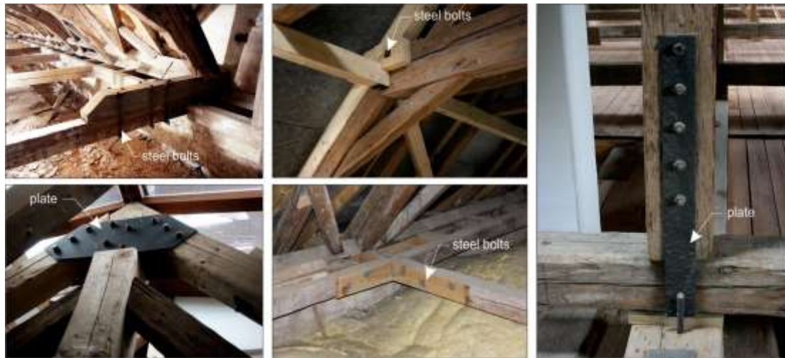
Fig 3. Traditional strengthening and stiffening of joints of roof truss members – using steel bolts and plates
