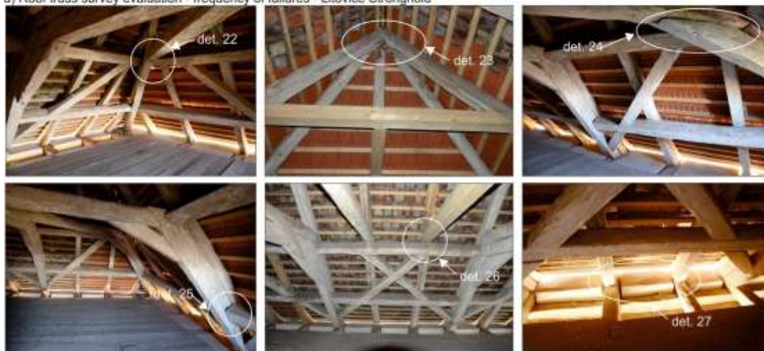
Fig 2. Roof truss survey evaluation – frequency of failures
