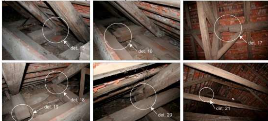
d) Roof truss survey evaluation - frequency of failures - Litovice Stronghold
