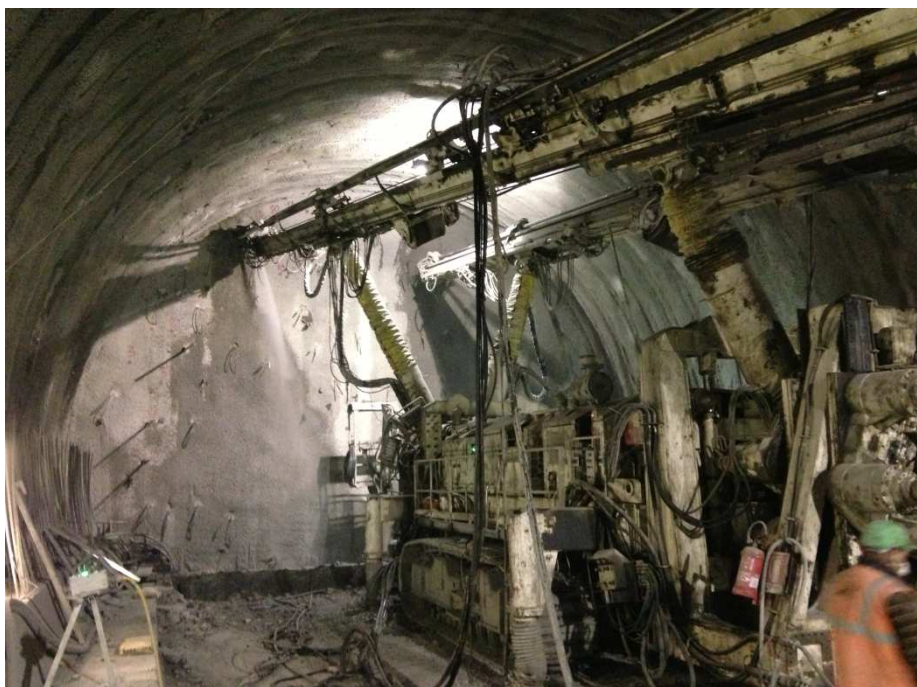
Fig. 1. Drilling of the tunnel face anchors, Val di Sambro Tunnel, Italy (author's archive)
