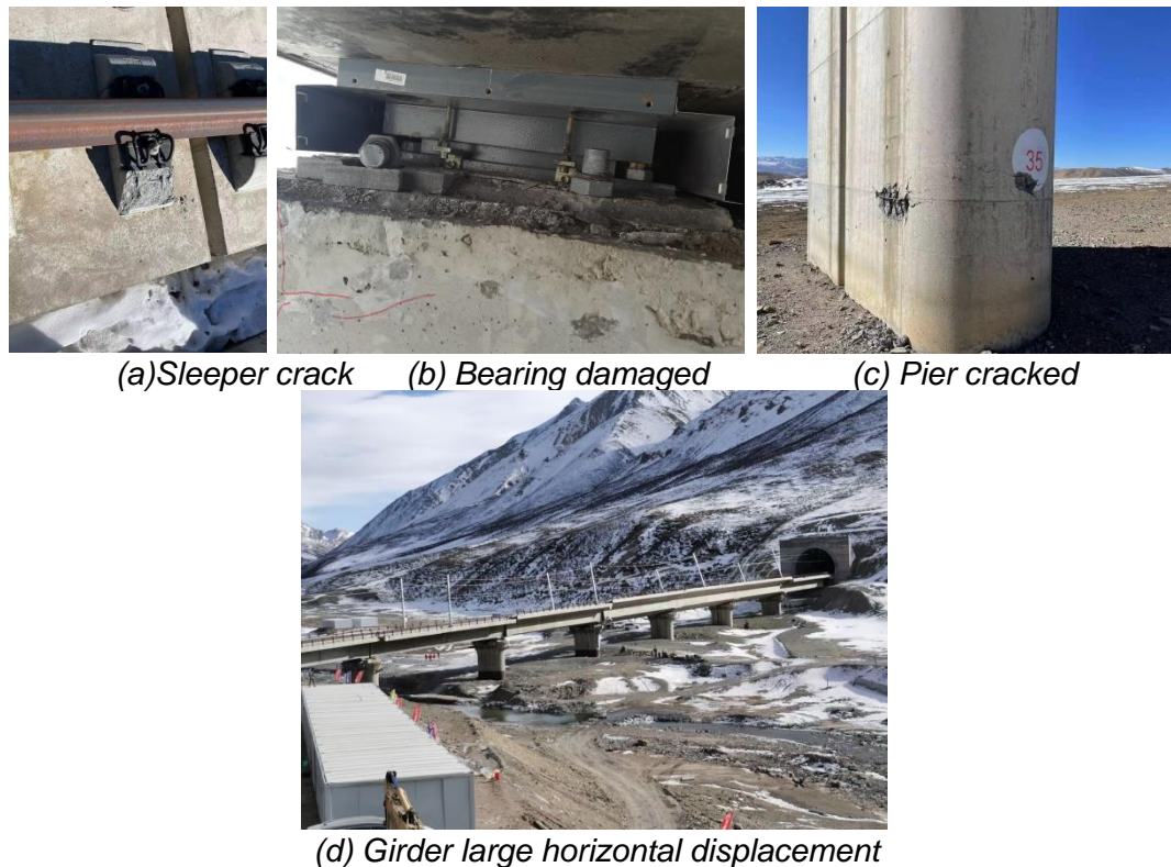
Fig.2 – Typical railway bridge seismic damage
