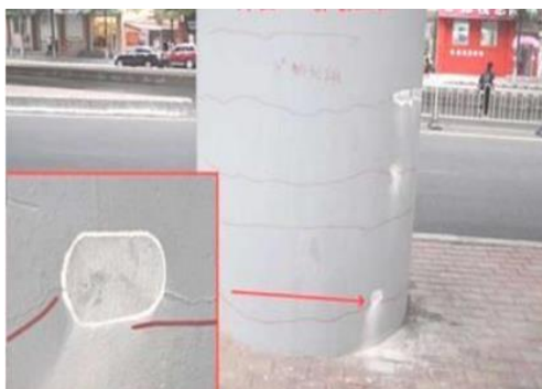
Fig. 8 – Bottom half-ring crack in bridge pier concrete
