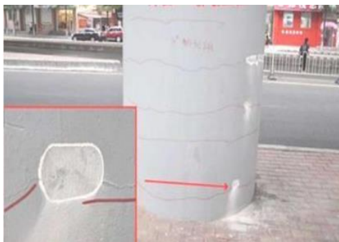
Fig. 8 – Bottom half-ring crack in bridge pier concrete
