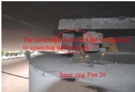
Fig. 6 – Compression deformation of lateral restraining steel bar
