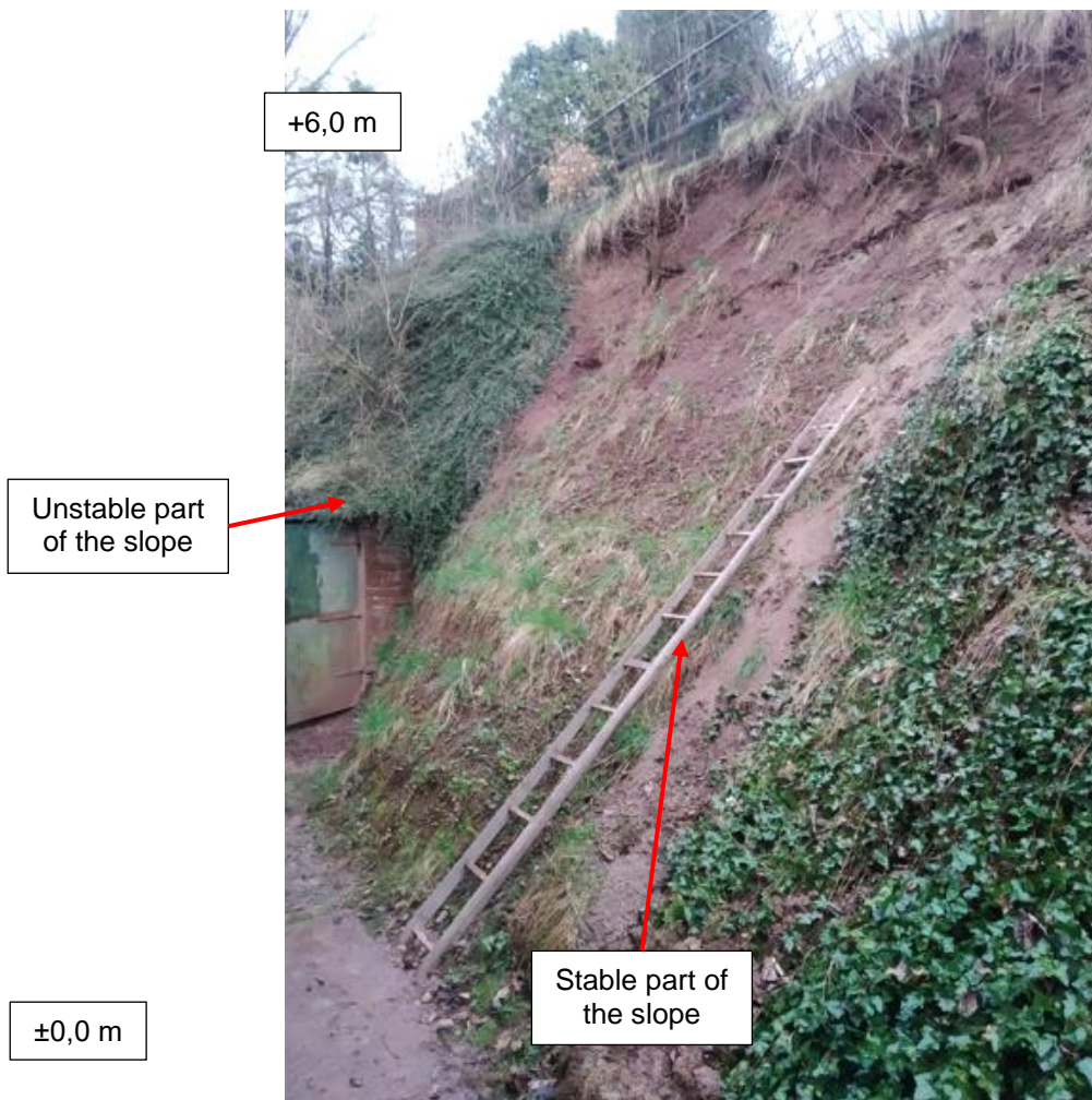
Fig. 1 - The cutting with the stable part covered with vegetation and the exposed unstable part
