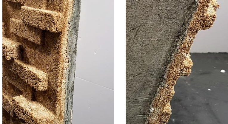
Fig. 10 - Detail view of the contact between two different concrete layers
